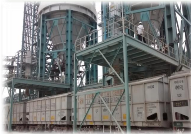
Dry Ash supply Rake Loading System
